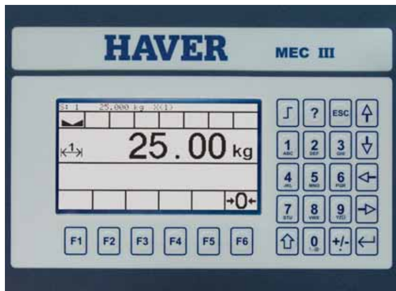
MEC III control terminal
